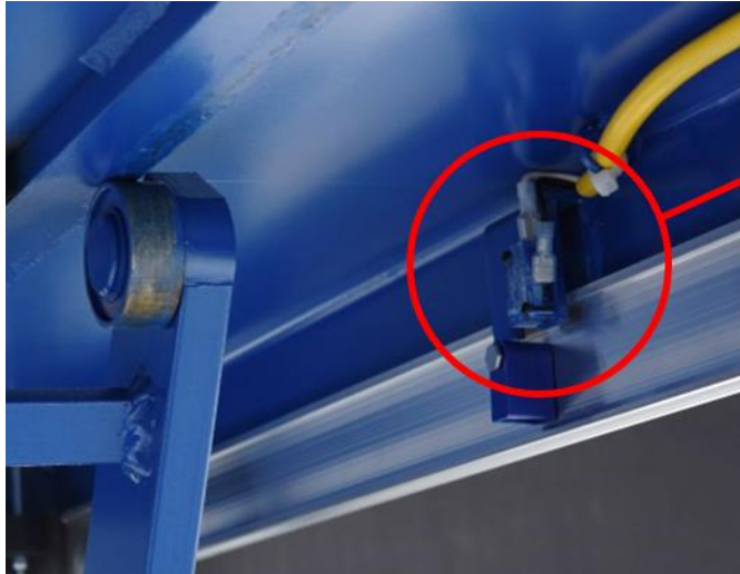
TOE GUARD LIMIT SWITCH (UNDER PLATFORM)
